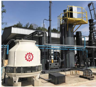
Waste Pyrolysis and Gasification ESP
