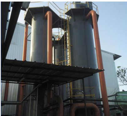
Biomass Gasification ESP
